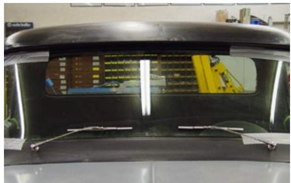
Photo 22. This photo shows the Wiper Arms and Blades installed on the truck.
